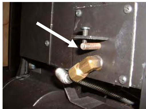
Photo 37 – Air Shutter Opened
