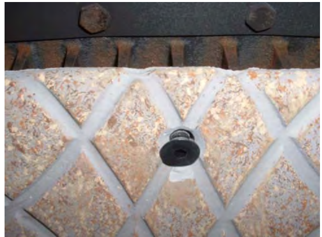
Photo 19 – Baffle Mounting Bolt
